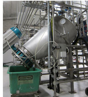
Impianto steam explosion
